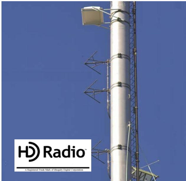
JHPC-2 +JHPC-HD-1 Separate Bays
