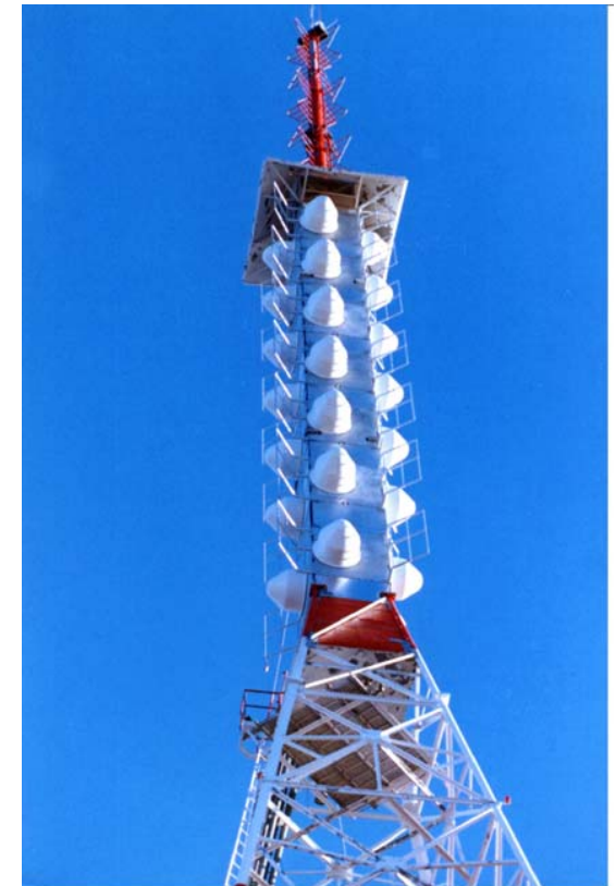
KSL - 13 Station FM Antenna
