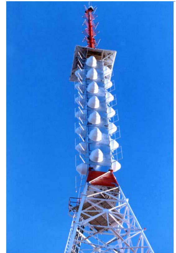
KSL - 13 Station FM Antenna
