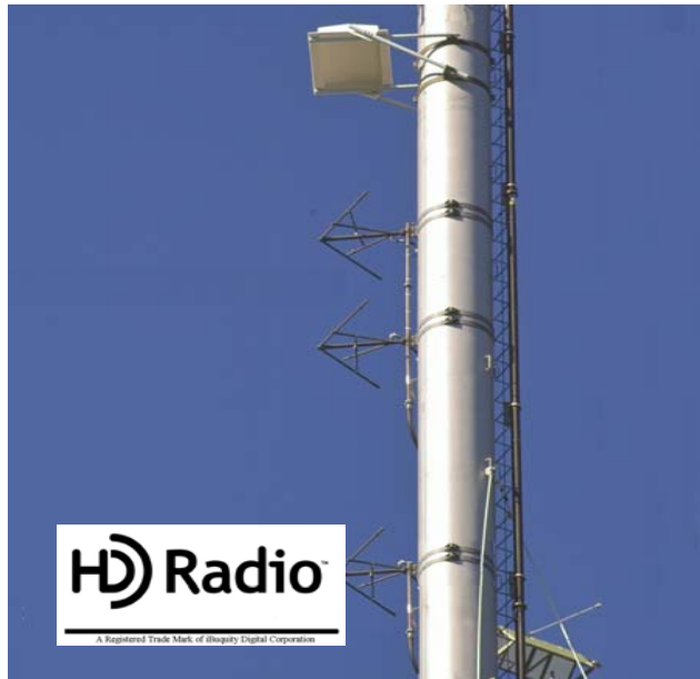
JHPC-2 +JHPC-HD-1 Separate Bays
